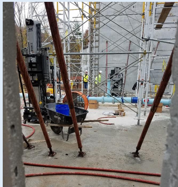
4 wall section braces keep each wall panel vertical until dome sectors are installed.
