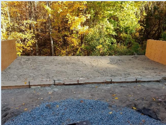
This is a concave up pouring bed for the 13 wall sections. Each wall section weighs 8.4 tons, is 4.5 inches thick, and Measures 12 feet wide by 24 feet high.
