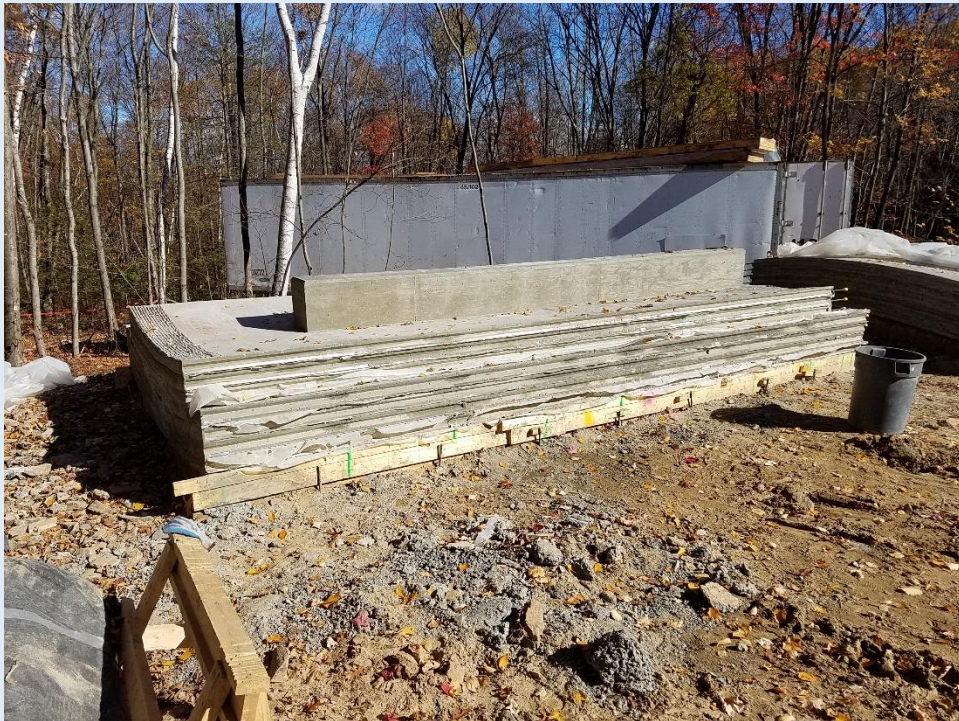
This top wall panel contains the iron "overflow" pipe, encased in concrete, to be used only if the pumps fail to turn off when the tank is full.
