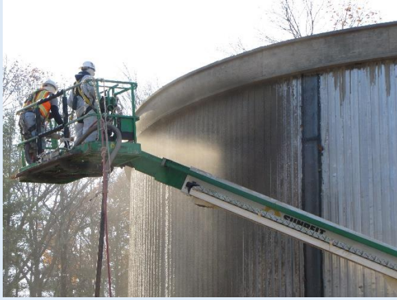
Dome ring (at top) in place, and “shotcrete” being sprayed on steel wall outer layer. Note bare steel on right, soon to be coated.
