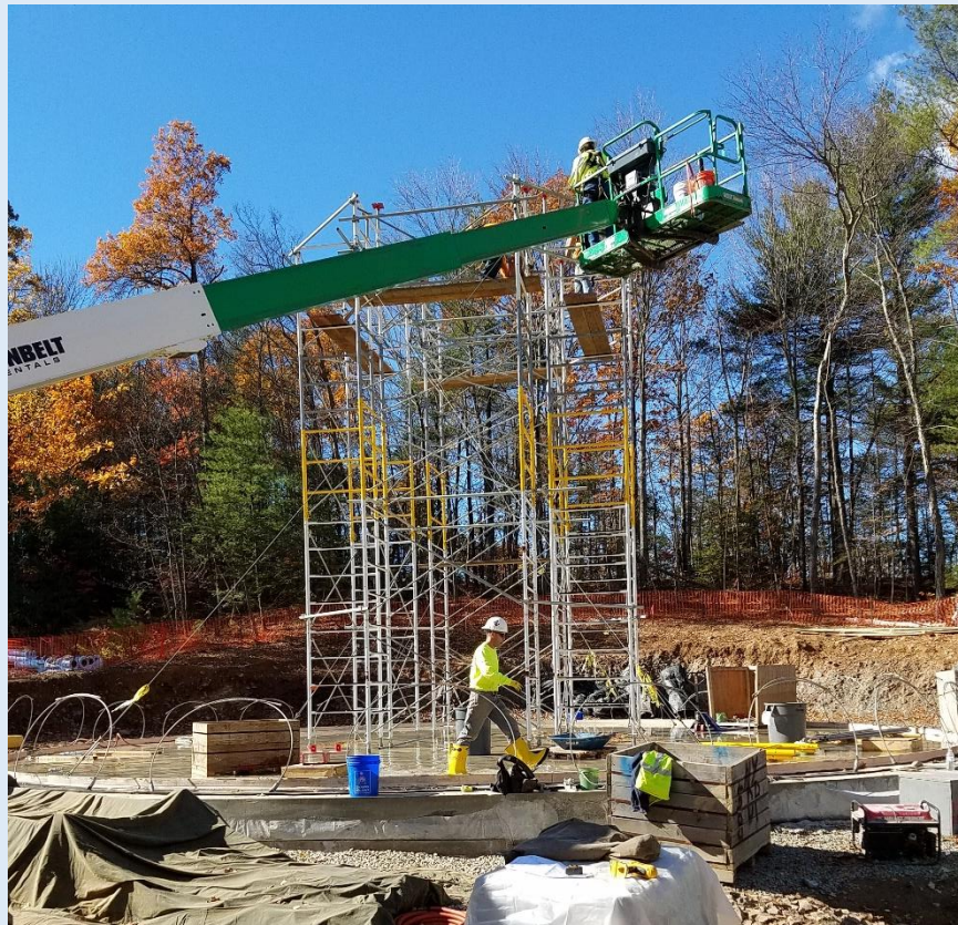
This scaffolding is temporary, used to hold the weight of the 12 “dome sectors” and one circular “dome panel” during the erection of wall panels and the dome.
