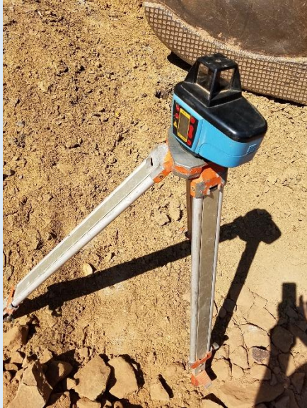
A laser level was used to ensure the new tank floor was level.
