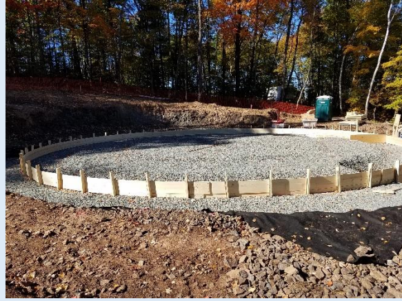
The forms for the concrete for the tank base are in place, and concrete trucks will soon arrive.
