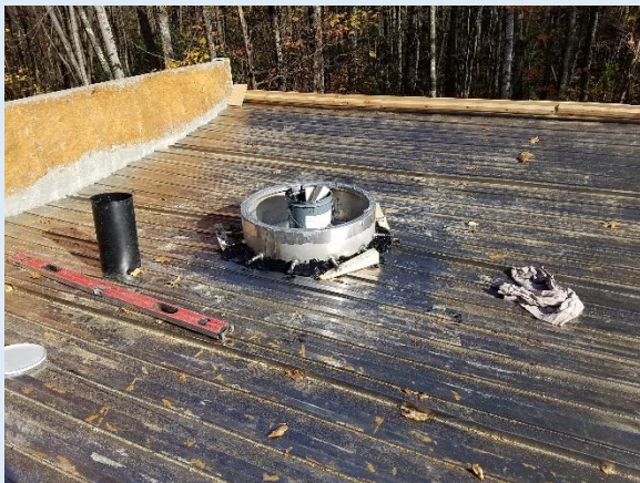
A 36" "manway" will allow entry into the empty tank.
