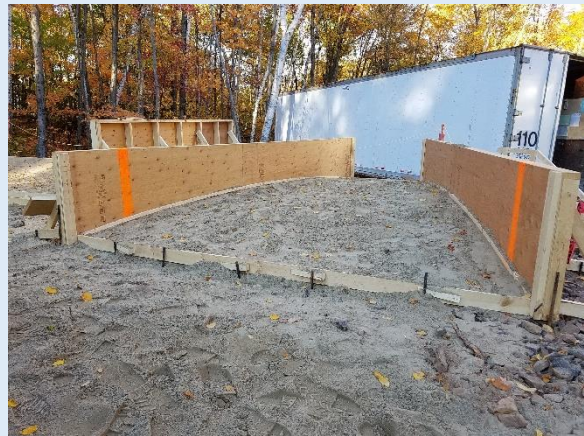
This is a convex up pouring bed for a dome sector. Each of the 12 dome sectors weighs 4.25 tons, is 17 feet long, 13 feet wide at wide end, and 4.5 feet at narrow end.
