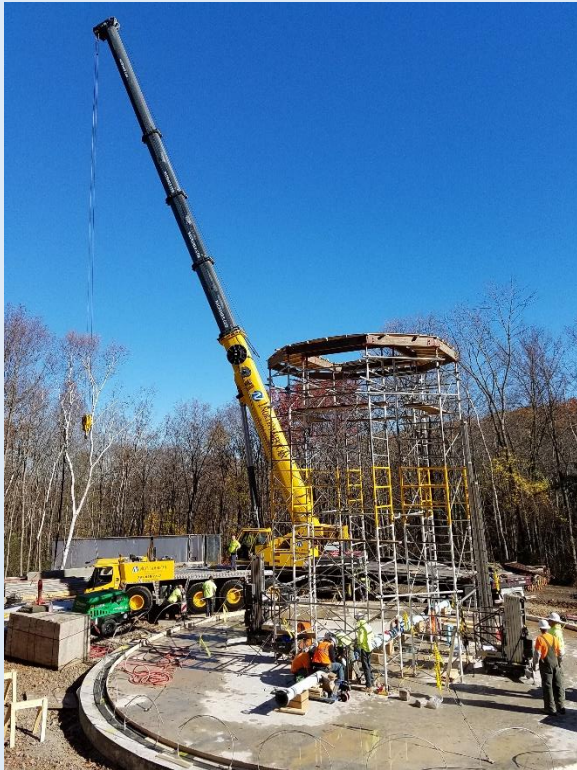
Scaffolding in place, awaiting dome panel. Done panel goes first, then wall panels.
