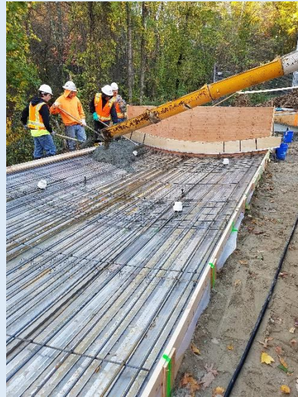
The pouring of concrete in the wall section 12' wide by 24 feet high is starting.
