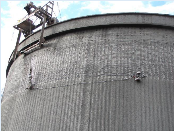
Apparatus used to wrap the tank walls with more than 400 turns of 0.168” steel wire. Here the top 8 feet or so of the tank has been wrapped with “pre-stress” steel wire.
