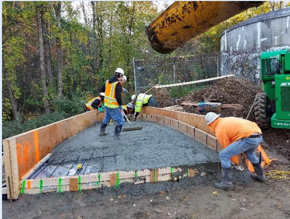
The rebar in the dome sector can be seen here as concrete is poured. The “screed board” on the right ensures the shape and thickness is correct.
