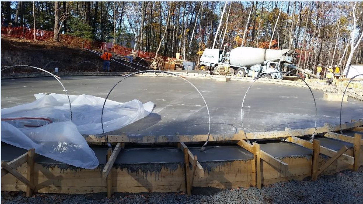
As of November 1, 2016, the concrete floor is complete. Next week a large crane will lift the wall panels into place, getting the tank closer to completion.
