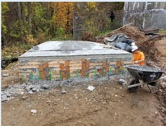
Roof dome sectors were poured one atop the other, one per day. 12 of these are needed, 4.25 tons each.
