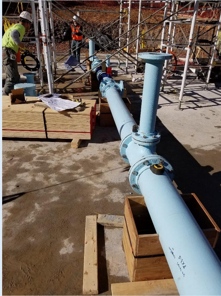
Inlet/outlet piping on floor of water tank. Passive mixing is used to prevent stagnation.
