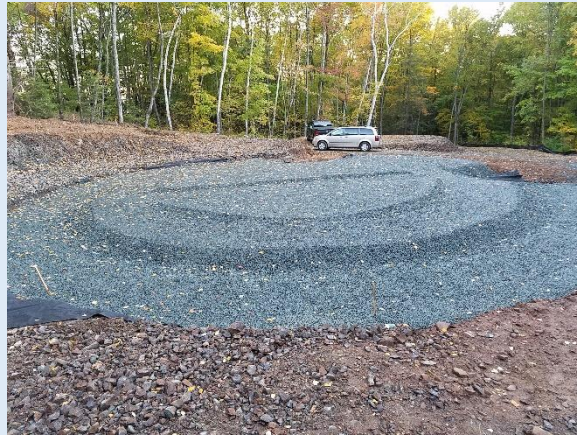
The site preparation is completed, ready for DN Tank company to begin construction.
