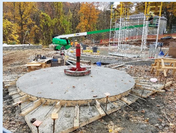
The center dome panel is curing. It will have the vent, and weighs 3.79 tons. The scaffolding that will support the roof dome sectors, and the center dome panel, during construction, can be seen being assembled.
