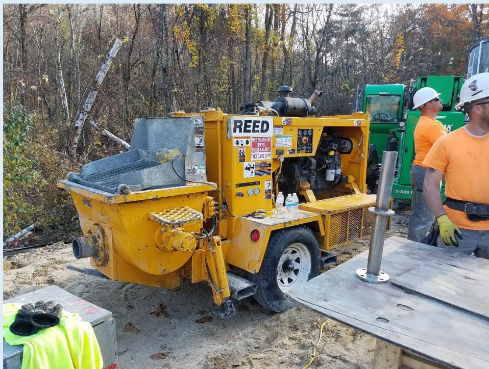
A concrete pump, to be used to bring concrete up to the top of the new tank to complete the connecting of the wall sections together, and the dome sectors together.
