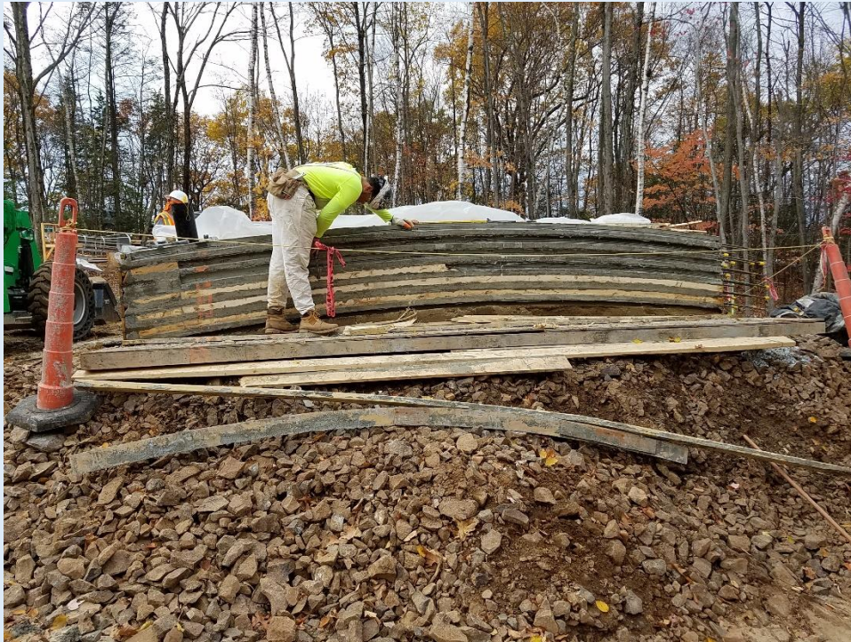
Six wall panels, one atop the other, were poured, one per day. The wood inserts which created the “keyway” at the bottom of each panel, are being removed above, prior to being lifted into place by a crane.
