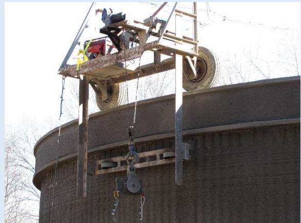
Close-up view of the wire wrapping “traveler dolly” that precisely spaces turns.
