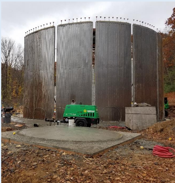
13 wall sections in place. Note the mold for circular dome panel in foreground.
